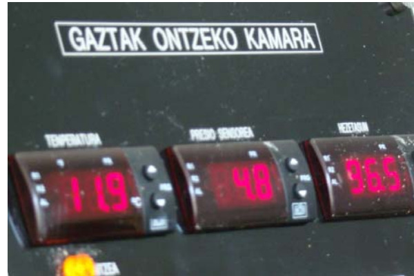
The control panel
